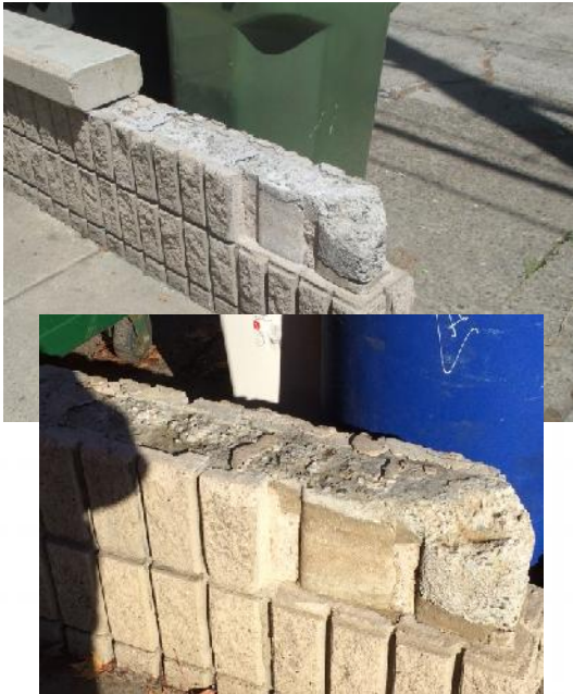
Before: Broken blocks, missing cap
